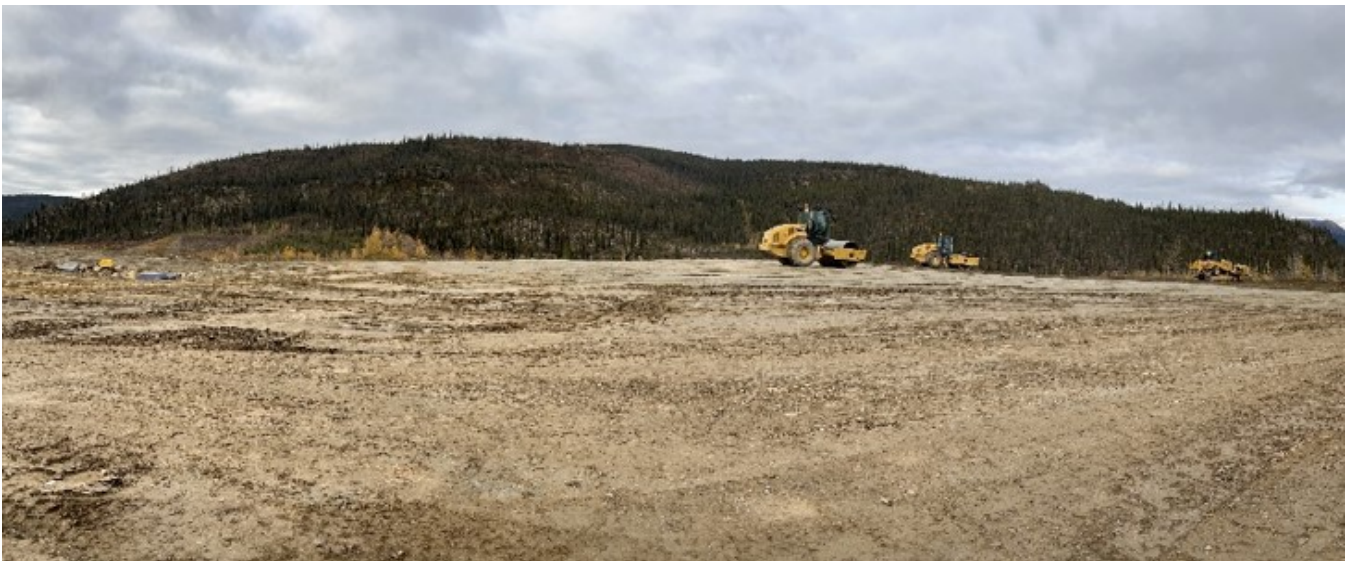
Progress on the preparation of the future camp area near the former freshwater reservoir dam. Photo courtesy of Parsons Inc.
