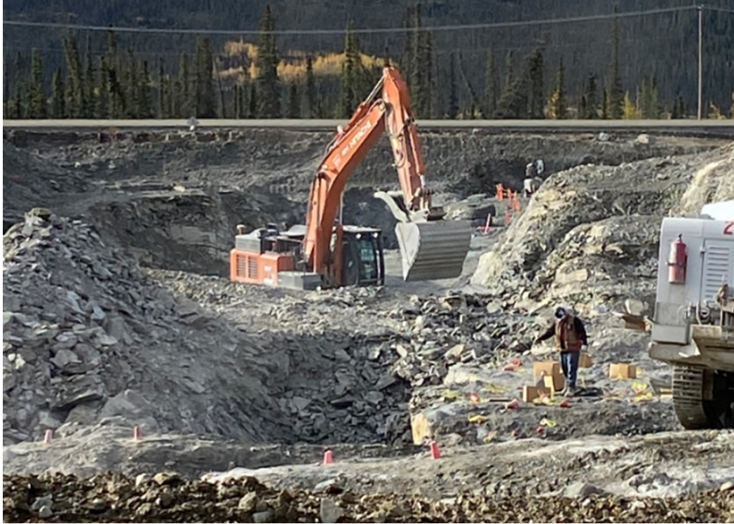
Excavation to prepare the footprint of the Permanent Water Treatment Plant. Photo courtesy of Parsons Inc.
