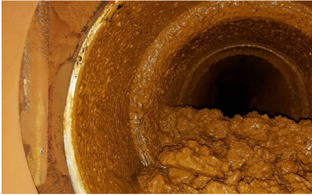
Inside the X13 pipeline during the cleaning work (pigging) in August 2023. Photo courtesy of Parsons Inc.
