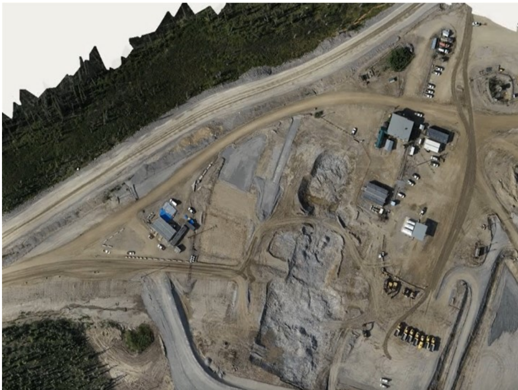
Progress on the Permanent Water Treatment Plant civil early works construction, August 2023. Photo courtesy of Parsons Inc.
